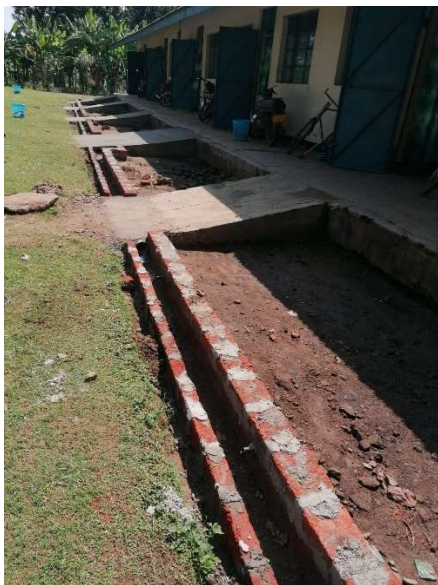
Men's side solving the drainage issue.
